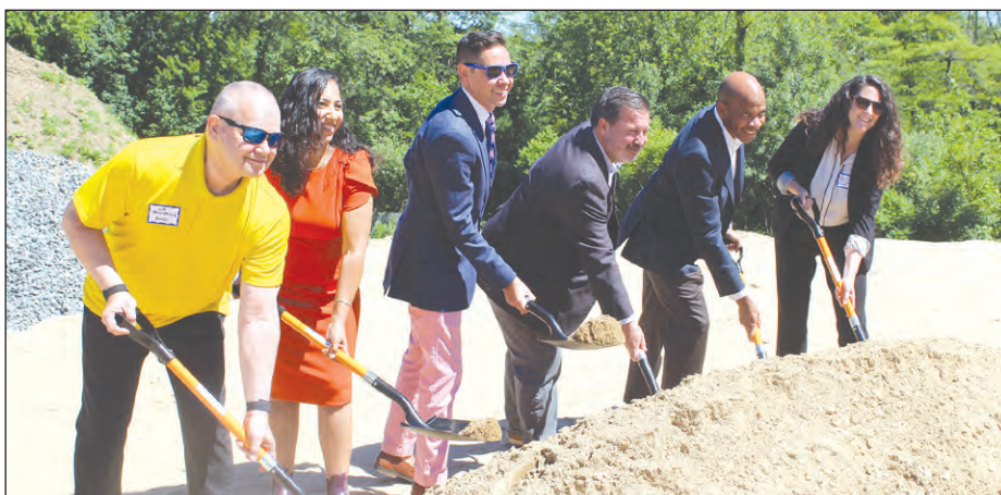
Speakers at the Friday morning ground-breaking tossed dirt on the pile as part of Greenstead Grove's ceremony.
