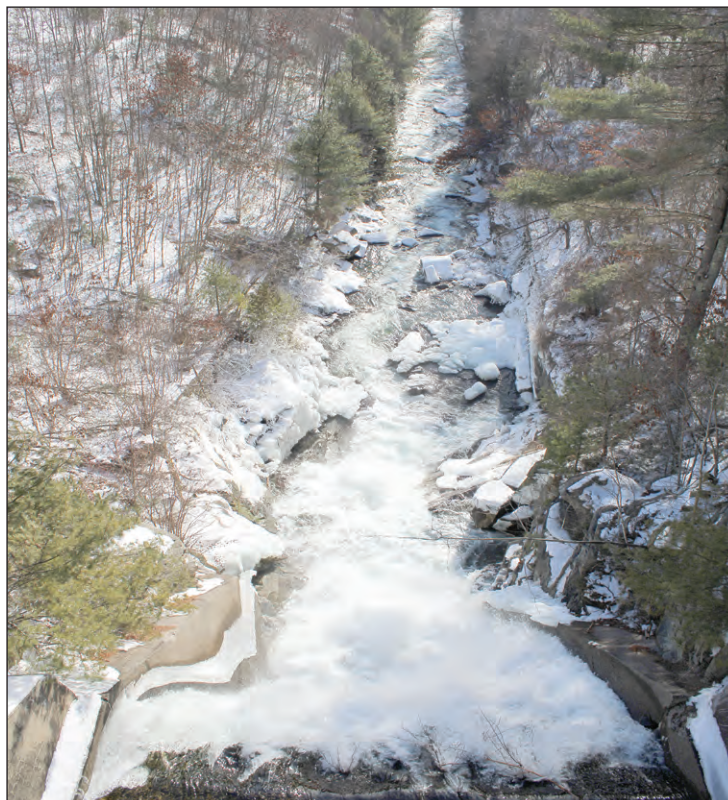
The lower spillway creates a waterfall, and only releases water when the Quabbin Reservoir is at or near capacity.
